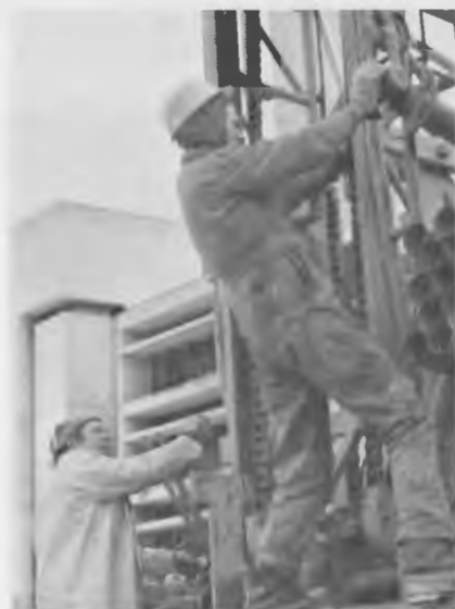
Workers from a private drilling company unload pipes from a rig prior to sinking of an aquifer well in the parking lot of AES building Downsview.
